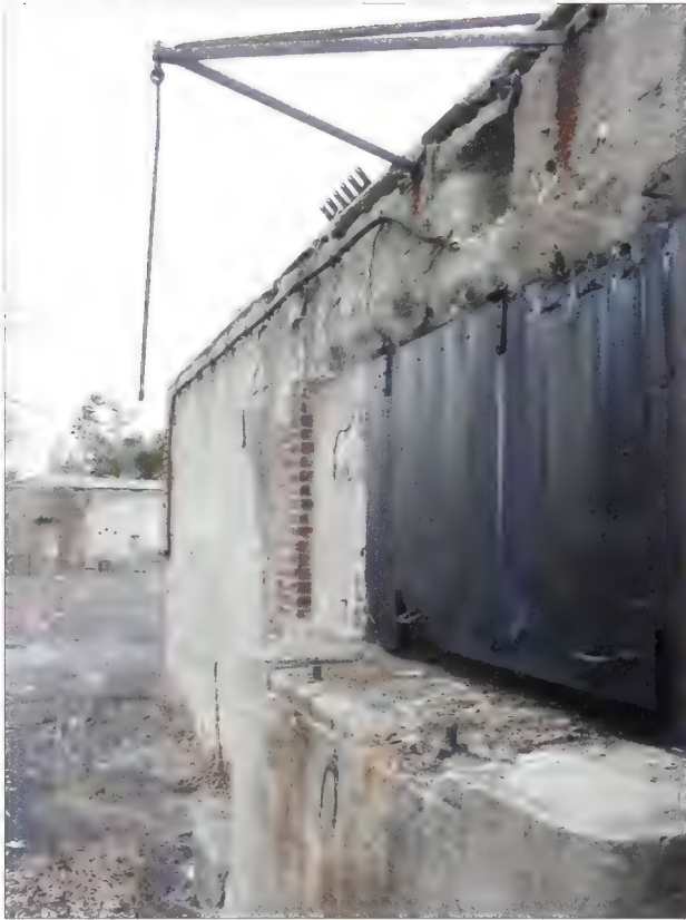
Figure 5.48. View of shell hoist metal door, Nine Gun Battery. Doors and windows should be properly mounted and locked to prevent unauthorized access. If a door is damaged or severely deteriorated, a new door should be fabricated to match the existing in materials and finish (Olmsted Center, January 2009).
